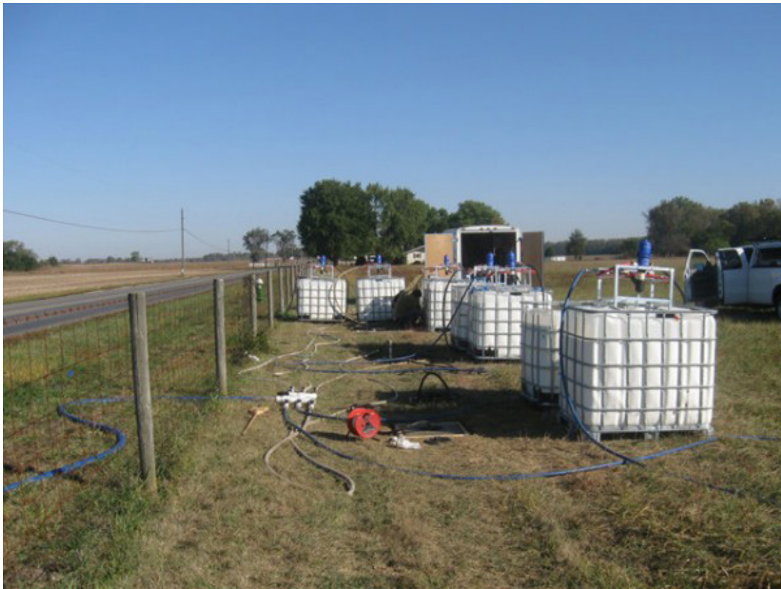
Figure 12. Example of an injection setup with EOS totes. Photo courtesy of Redox Tech.
