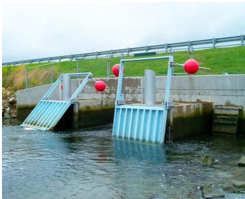
Figure 19: Representative photo of self-regulating tide gates from location (Waterman Industries).
