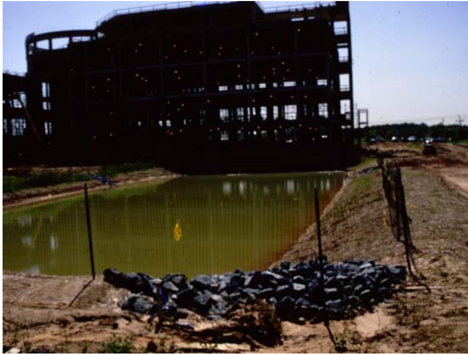
Typical example of a sediment trap used during the construction of a commercial office park (Source: CWP, 2001)
