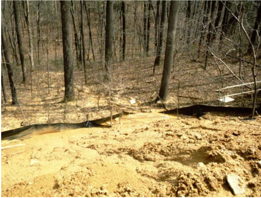
An improperly sited and poorly maintained silt fence (top) versus a super silt fence reinforced by chain link fencing (both) (Source: CWP, 2001)
