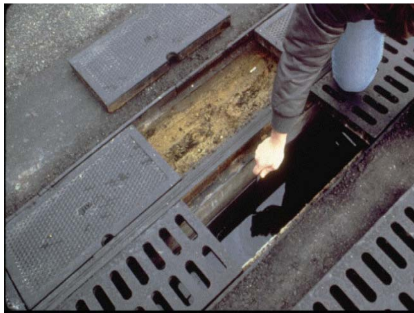
Example of perimeter sand filter (Source: MDE, 1999)
